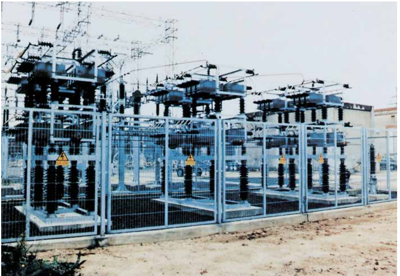
36 MVar - 110 kV - 50 Hz
