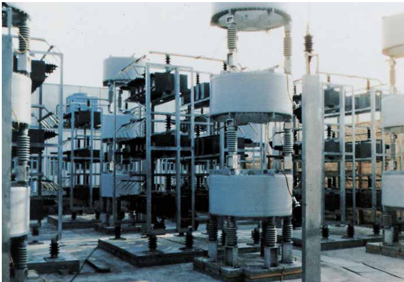
2 x 19,5 MVar - 22,7 kV - 3rd - 4th harmonics
