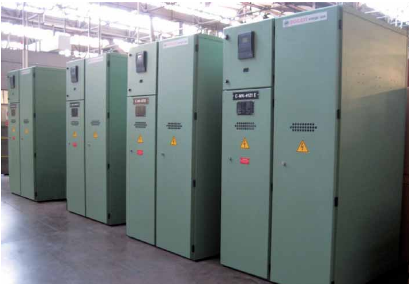
2 MVar - 12 kV - 50 Hz - PFC panels with switch and inrush current limiting reactors
